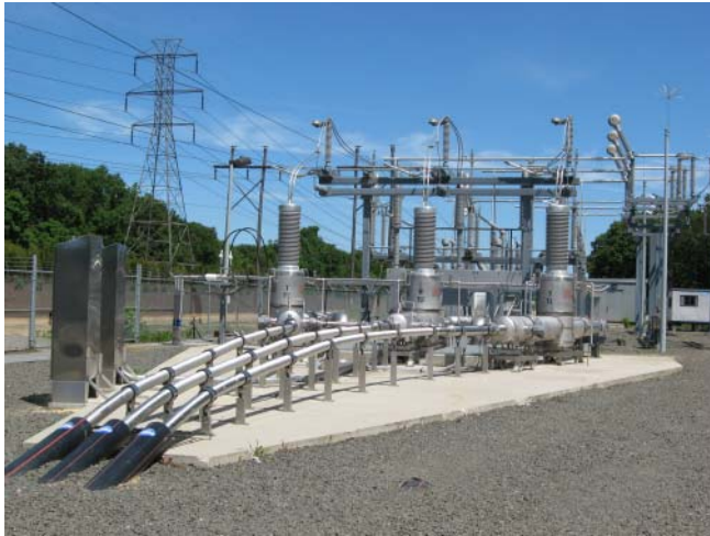
Fig. 8. LIPA HTS cable project (Courtesy of AMSC).
