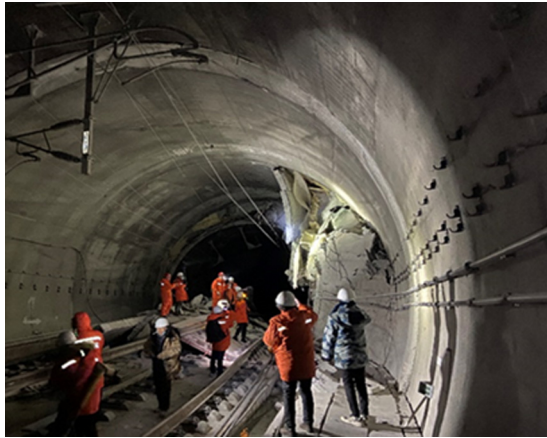
Figure 1: Damages caused by faults in the Daliang Tunnel.
