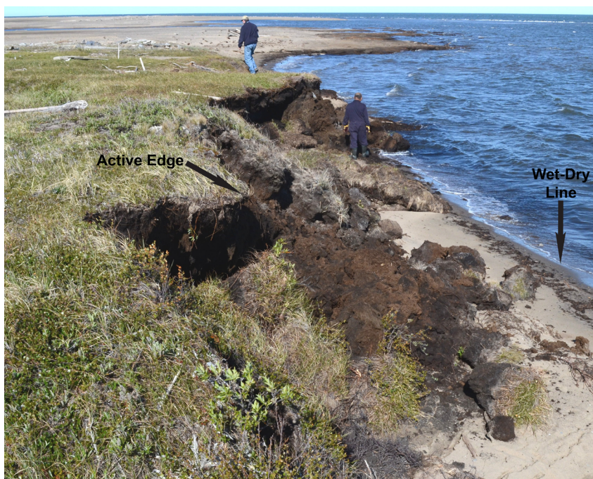
Fig. 6: Eroding shoreline near monitoring stakes at Toker Point.
