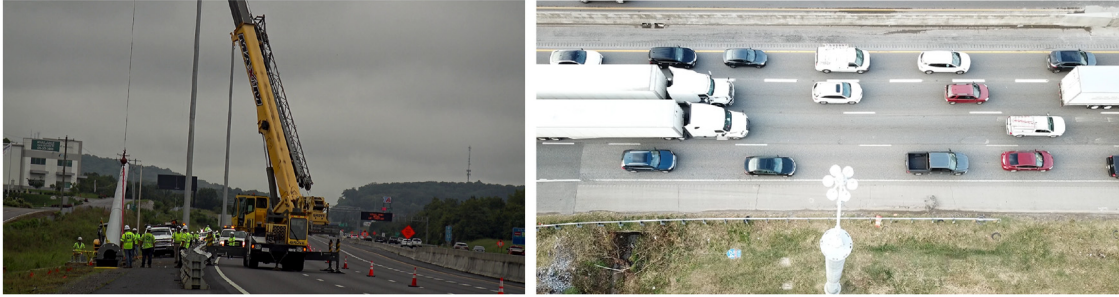
Figure 9: Left: Installation of a roadside pole. Right: aerial view of the installed pole with 8 cameras and I-24 traffic underneath.
