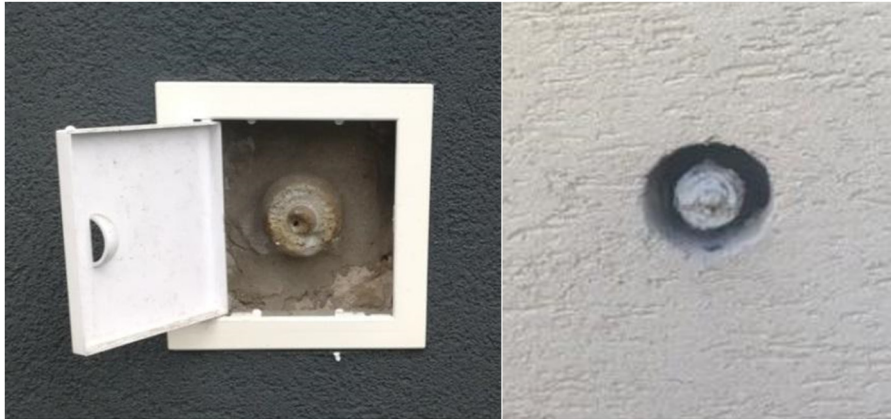
Figure 13: Points built-up in incorrect manner.
