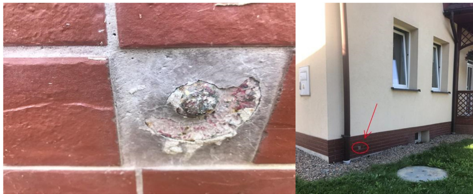
Figure 14: Photographs of the destroyed point – T point location zone.
