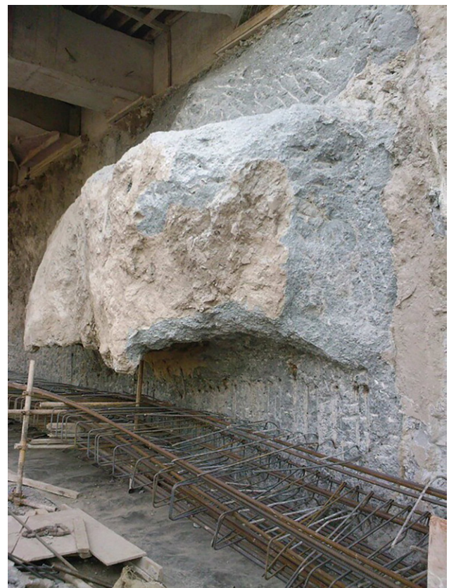
Figure 1: Concrete overflow caused by local failure of a slurry trench.
