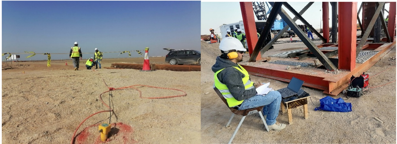
Figure 11: Vibration monitoring system.
