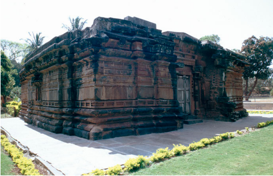
Plate 5.45: The complete shrine section of the Cikka Basadi at Belgaum has been demolished. The debris has been removed and what remains of the jinālaya has been sealed off with a door.
