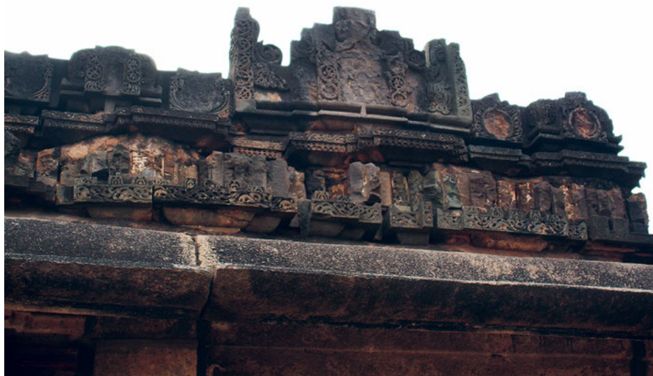
Plate 4.13: Destruction of Jaina images and decorations on the parapet of Lakṣmeśvara Temple (Gadag District), detail.
