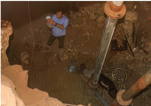
Inside the pumping station in Shaikh Hadeed in Iraq, the only window to the habitat of Caecocypris basimi and Garra widdowsoni . © O. F. Al-Sheikhly.
