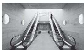
226 CAELA LIGHTING SYSTEM
